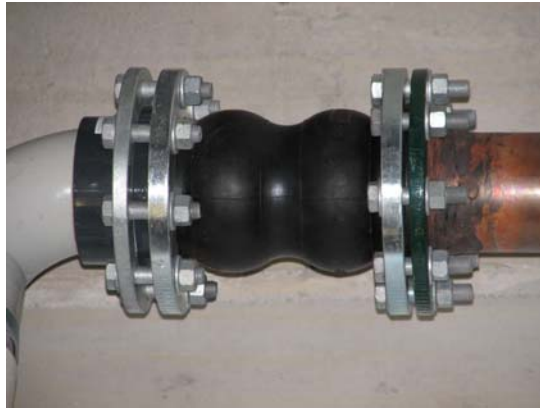
Figure 8.11 piping system connection in seismic zone utilized in Hospital project in Wellington, New Zealand, (Three center field mission - August 2006)
